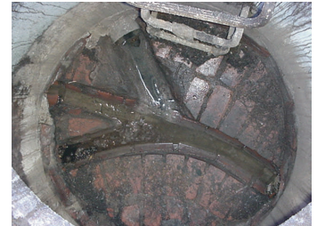
Free flowing sewer line.
