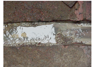
Sewer line clogged by grease blockage.
